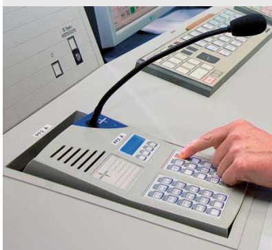
30 DTM 010 installed into a control desk
